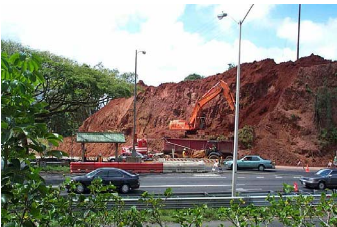
Work to repair the hillside along Kalanianaʻole Highway at Castle Junction began in January 2004 and is expected to be completed by December 2004. The landslide caused by the heavy rains in the summer of 2003 left one Honolulu-bound lane completely closed for several months.
