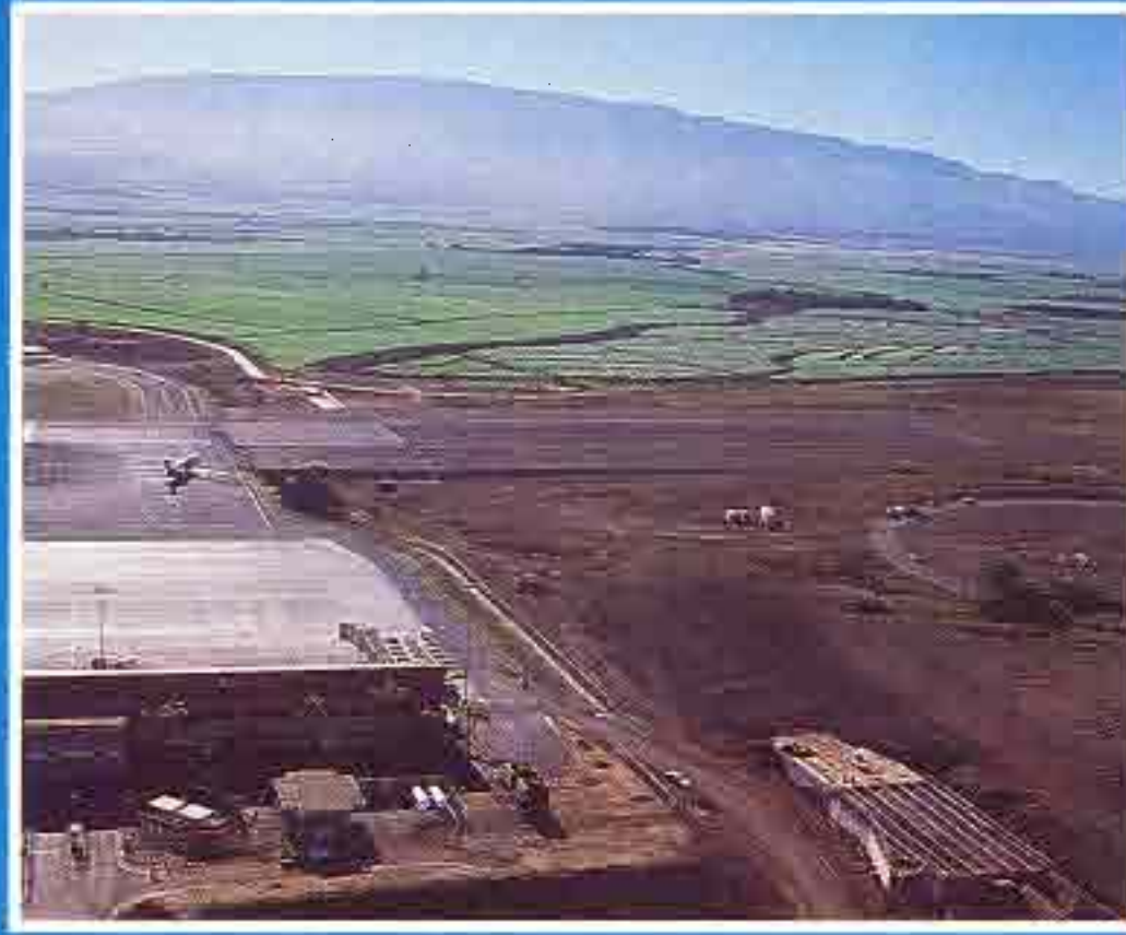
Construction on Kahului Airport runway safety area is scheduled to be completed in December 1990.
